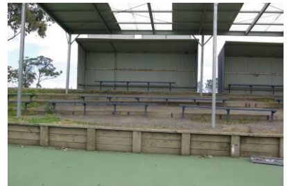
Tiered seating area (on bank) – no balustrades as retaining wall to courts from banks appears higher than 600-700mm. No ramp access to courts.
