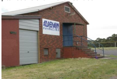
Football Oval Pavilion – no internal inspection as access was restricted. External access appears not compliant to current BCA / DDA requirements.
