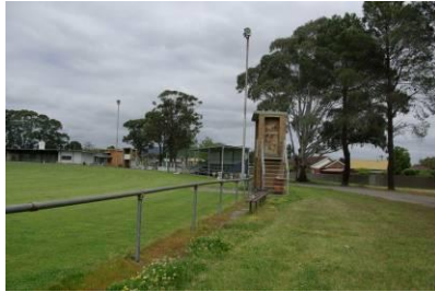
Boundary fencing and existing sport lighting towers appear 'tired' and have evidence of corrosion.
