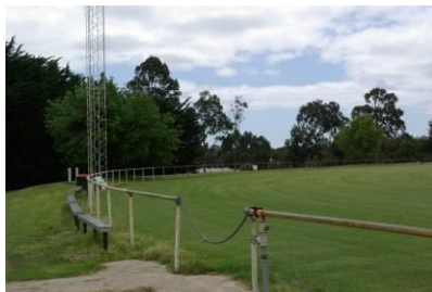
Boundary fencing and existing sport lighting towers appear 'tired' and have evidence of corrosion.
