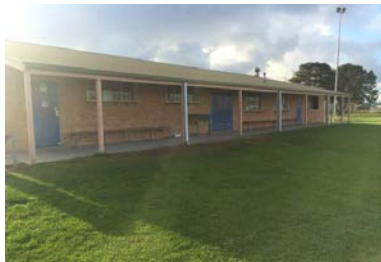
Overall the sports pavilion is in a good condition. Opportunity to refurbish and construct second storey.
