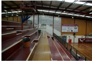
Seating plats appear too narrow and too high. Main circulation path (centre) should be provided a handrail to minimise any fall risk. Balustrade to edge not compliant – appears to be less than 1.0m in height. Also can be climbable.
