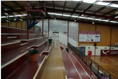
Seating plats appear too narrow and too high. Main circulation path (centre) should be provided a handrail to minimise any fall risk. Balustrade to edge not compliant – appears to be less than 1.0m in height. Also can be climbable.
