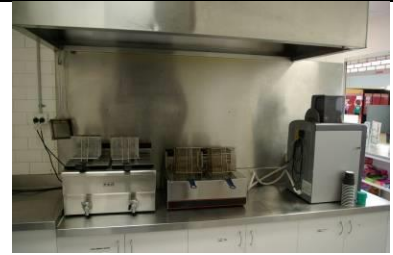
Kiosk – main cooking area appears not to current BCA requirements. Joinery units under fryers appear a potential fire hazard and Main exhaust appears reasonable with height and overhang from wall.
