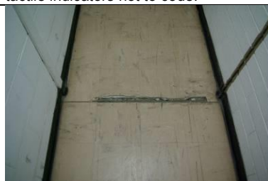
Main circulation hall to change rooms is too narrow (less than 1350mm), not ideal for 2-way traffic and flooring in poor condition. Potential trip hazards evident.
