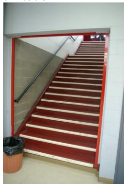
Stair access to additional courts seating areas not compliant to current BCA/DDA standards. Handrails and tactile indicators not to code.
