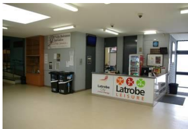
Main entry, control / reception counter. Counter not catering for wheel chair access by patron/ player.
