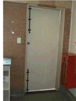
Image 12: Main egress door from kitchen not compliant to current BCA regulations.
