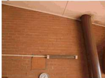
Image 7: Water damage to ceiling and internal cracking to masonry wall.
