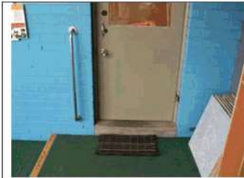
Image 7: Step entry into the pre-school children's amenity area – not accessible. Recommend to install a ramp threshold. Door hardware not compliant for an exit/egress door.
