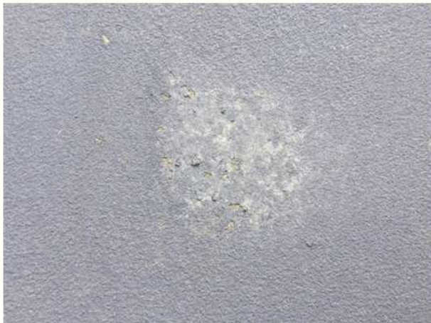
Isolated surface failure. Faded acrylic with very small areas of delamination within it.
