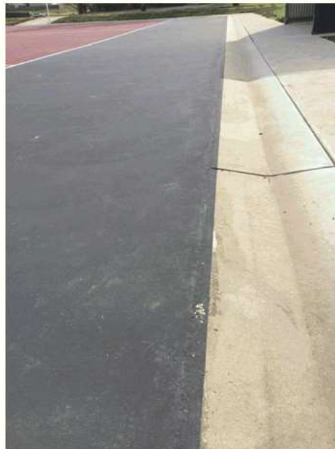
Smaller sections of delamination along the Eastern boundary of Courts 5-10.
