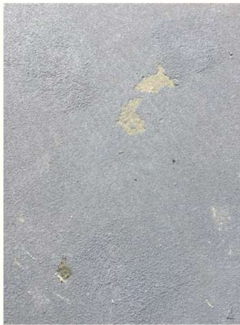
Delamination area on the Court 5-10 pavement. The Qualipur Stain Block product is visible and intact.
