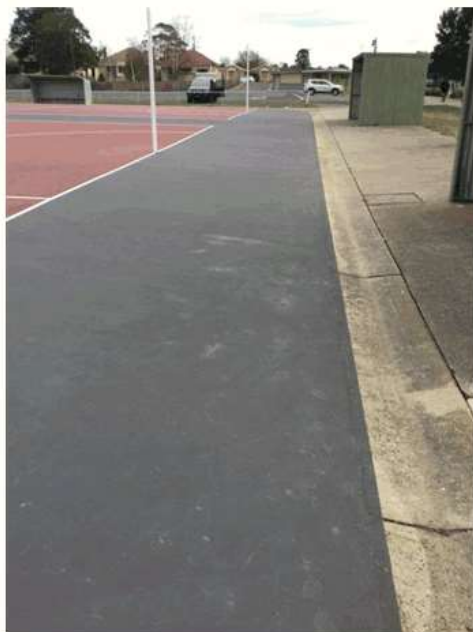
The gradient along the Court 5-10 Northern boundary appears steeper than the 1% fall recommended.
