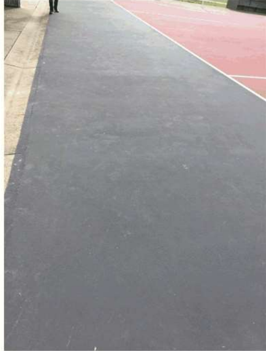
Delaminated areas along the Court 5 Western sideline.
