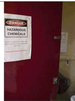
Image 15: Latch to door not acceptable to unisex toilet as an occupant can be locked within room.
