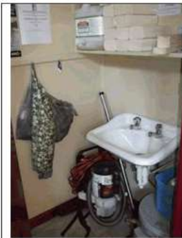
Image 13: Unisex toilet combined cleaner's room not really acceptable. Hot water unit (exposed) under the staff basin may be considered a hazard to health. (Young fingers may get burnt from the excess heat of unit and exposed piping.)
