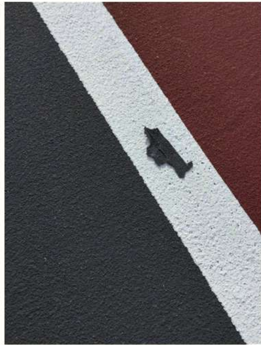
Piece of delaminated acrylic sitting on the court surface. The sample confirms that the delamination has not affected the Qualipur.
