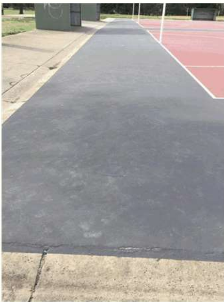
Patched areas in the North West corner of Court 5. View along the Northern pavement boundary shows increased gradient fall.
