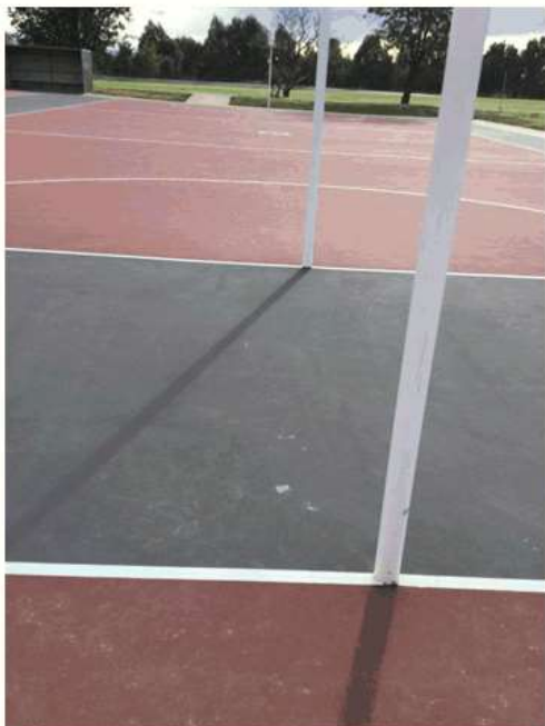
Delamination area between Courts 7&10. The Qualipur Stain Block product is visible and intact.
