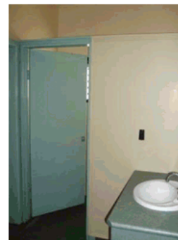
Image 3: Toilet partition may contain asbestos. Due to age of facility it's most likely unless refurbished in the past 20 years.
