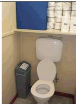
Image 14: Unisex toilet. It is not recommended that a shelving unit is located at the height of an adults head while seated. Ideally the storage of goods is not recommended within an amenity facility.
