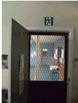
Image 8: Entry / exit door not compliant to BCA regulations. Note – existing exit sign not compliant. Requires to be illuminated.
