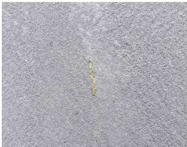
Delamination area between Courts 3&4. The Qualipur Stain Block product is visible and intact.
