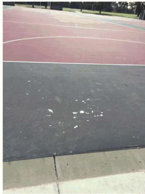
Large delaminated area to the South of Court 9.
