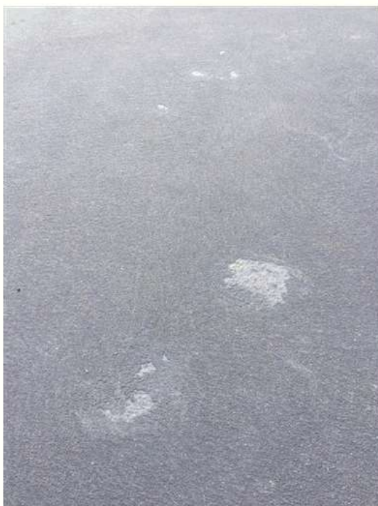
Single coated delaminated areas between courts 7&10
