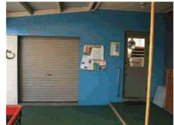
Image 12: External entry to storeroom via roller door to play equipment store room.
