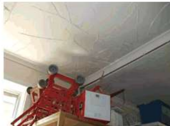
Image 10: Main store room – location of some equipment not readily accessible and issues with working at height to store equipment. Store room may require a better storage solution or more room. Water damage apparent to ceiling lining.
