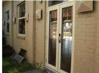
Image 10: Western Door (egress) to be confirmed. No accessible path from this door to main foot path. Also exit doors within 6.0m of adjoining building – no evident fire rating.
