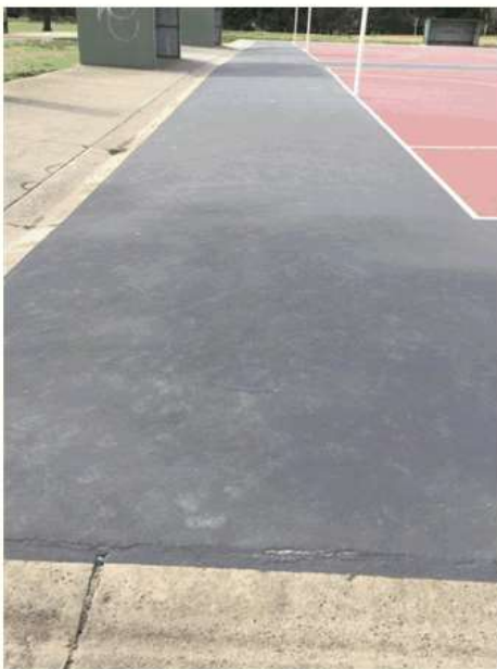
Patched areas in the North West corner of Court 5. View along the Northern pavement boundary shows increased gradient fall.
