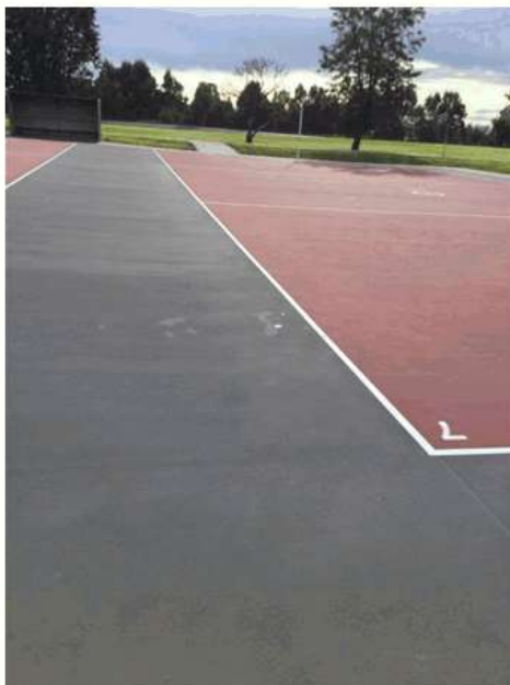
The area between Courts 6&7 – showing a mixture of patched and new delamination.
