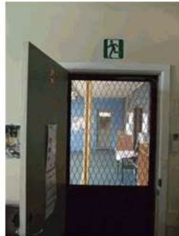
Image 8: Entry / exit door not compliant to BCA regulations. Note – existing exit sign not compliant. Requires to be illuminated.
