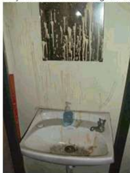
Image 14: Back of house amenities very poor. Require a general clean or refurbishment. Unisex room not complaint for ambulant users.
