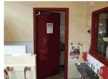
Image 12: Staff / Parent uni-sex amenity for pre-school is off the children's amenity area. Not really acceptable. Unisex amenity area is also the cleaner's room. Again not acceptable.
