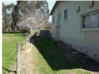
Image 7: Exterior of building within 6 metres of boundary. Under the current BCA this wall may be required to be fire rated.
