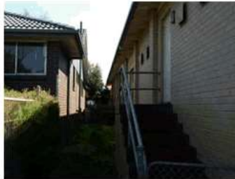
Image 8: Exterior of building within 6 metres of adjoining pre-school. Under the current BCA these walls may be required to be fire rated. Door Egress from Hall not compliant to BCA regulations. Landing to stairs not big enough and no dedicated pathway from exit to main foot path.
