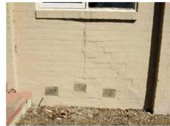
Image 6: Structural cracking to both brick and mortar joints. Evidence of building settlement. No evidence of brick construction / expansion joints along the eastern façade.
