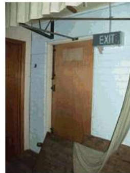
Image 15: Back of house exit blocked. Door hardware not compliant for an exit door.
