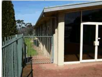
Image 11: Child proof gate from main courtyard to grade ramp (egress). Ramp is not BCA compliant due to grade (fall) of ramp and handrail.
