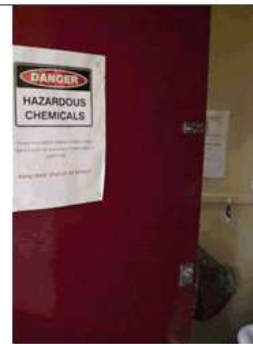
Image 15: Latch to door not acceptable to unisex toilet as an occupant can be locked within room.
