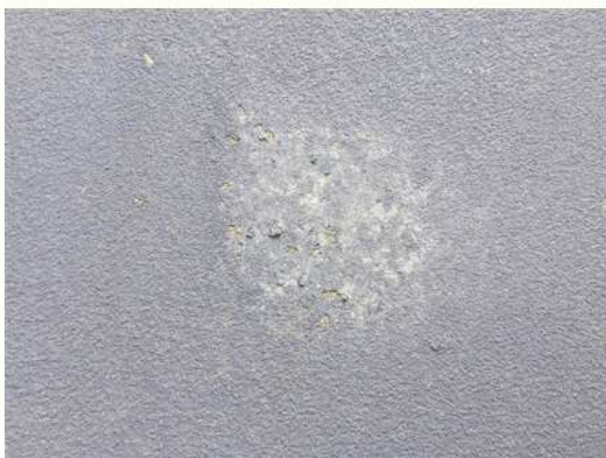
Isolated surface failure. Faded acrylic with very small areas of delamination within it.
