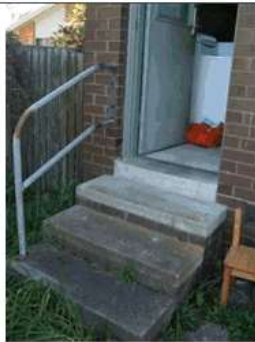
Image 8: Access to southern exterior area/ garden is via steps in staff kitchen. Doorway too narrow to current BCA / DDA opening clearance – under 850mm. No step landing to steps at door way. Handrail not compliant.
