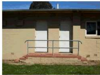
Image 4: Existing egress doors from storage room and kitchen. Door landing and steps not compliant to current BCA egress requirements. No concrete path from steps. Clearance too small from door ways.
