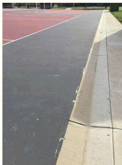
Delaminated areas along the Eastern sideline boundary of Courts 7&10.
