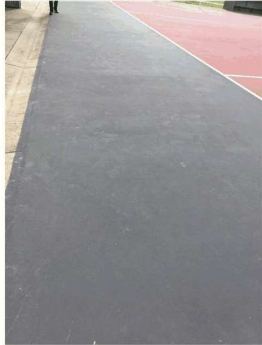
Delaminated areas along the Court 5 Western sideline.
