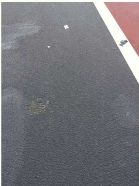
Close up of delaminated acrylic area between Courts 6&7 shows the glossy Qualipur Primer underneath.
