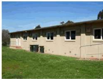
Image 5: side façade along memorial hall. No pathways from egress ramp, and exit doors to main road and foot path.
