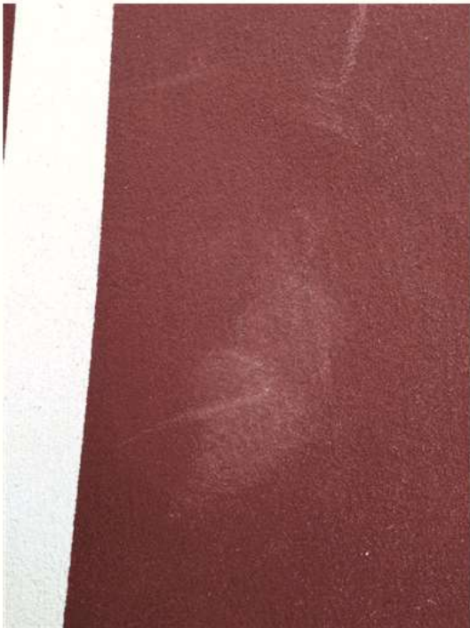
Example of faded acrylic colour where light scuffing has occurred. Sand is sitting freely on the surface.
