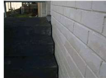
Image 9: Western egress steps not structurally sound as they are not connected to the main building.
