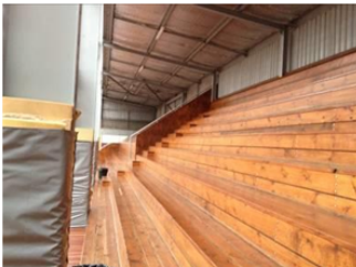
Timber tiered seating – too steep. May be considered not compliant to current BCA & DDA regulations.
