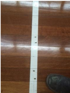
Stadium 1 - Nails protruding from main sports floor in Court 1. Not safe. Should be rectified immediately.
