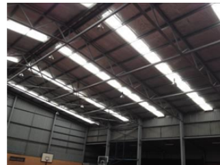
Stadium 2 + 3 – roof leaks in areas. Leaking may be due to expansion joints or construction junction between skylight and main roof sheeting.
