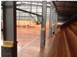
Safety run-off zone between courts, columns and seating too narrow. Pedestrian gap between seating and columns non-existent. Padding to wrap around columns and not just playing side.
