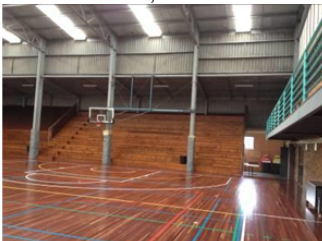
Stadium 2 +3 – main spectator seating obstructed with existing steel columns. Also seating located at end of courts – not ideal.
