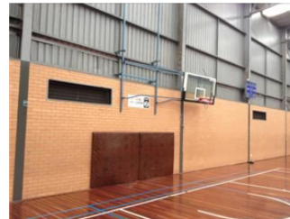
Not enough padding to goal end of courts 2 + 3. Padding should extend the length of the goal zone for netball and not just cater for the basketball key. Also not enough safety run off for both basketball (2.0m) and netball (3.05m)
