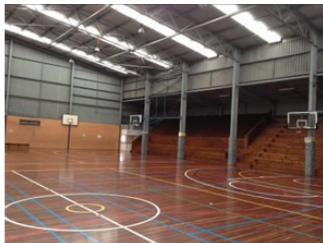
Stadium 2 +3 – main spectator seating obstructed with existing steel columns. Seating needs to extend along court 3. Courts are multi-line – sometime difficult to determine which court playing on.
