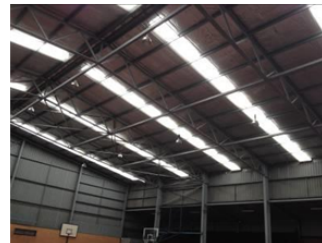
Stadium 2 + 3 – roof leaks in areas. Leaking may be due to expansion joints or construction junction between skylight and main roof sheeting.
