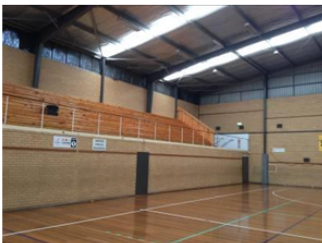
Seating to Court 1 is via elevated walkway from Court 2. Height of tiered seating appears reasonable to BCA, however did not observe any wheel chair dedicated seating zones (compliance to BCA and AS 1428)
