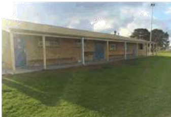
Overall the sports pavilion is in a good condition. Opportunity to refurbish and construct second storey.
