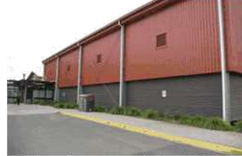
Existing show court exterior. Sub floor venting is restrictive due to levels of landscaping and entry path.
