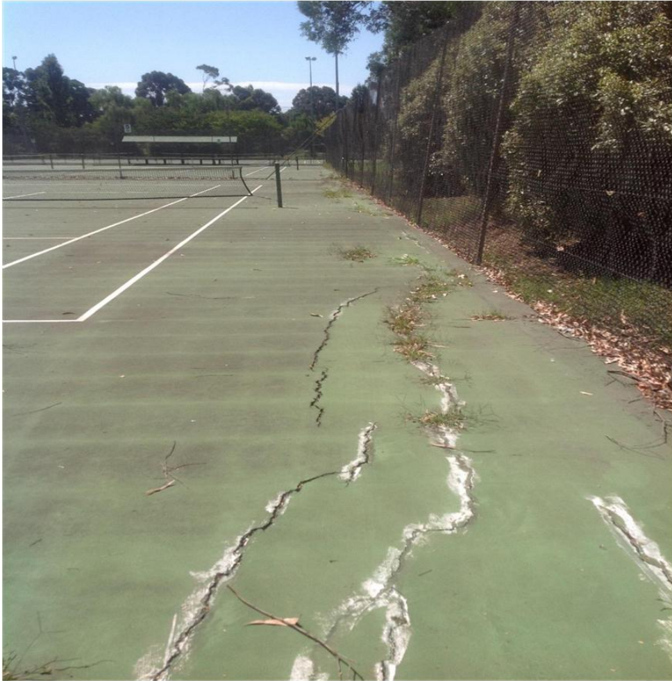
Immediately adjacent to a stand of trees and shrubs, the pavement has collapsed and can no longer be patched up.
