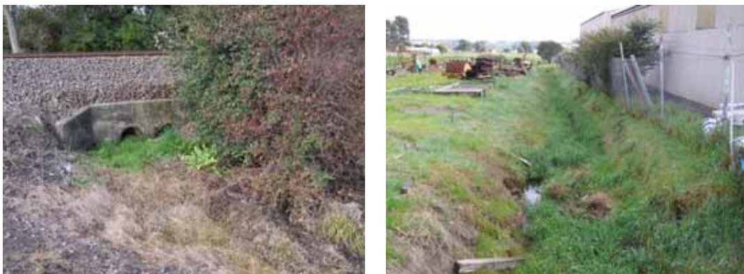
Photos 7 and 8 One set of Waterloo Drain culverts under Railway and downstream of Waterloo Road at W4 Industries
