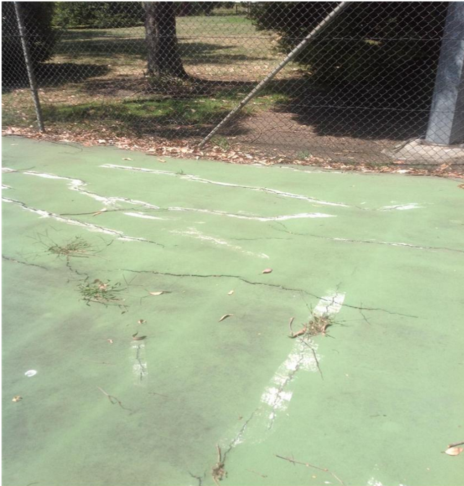
Evidence of past crack repair attempts and further new cracking throughout the court can be seen above.
