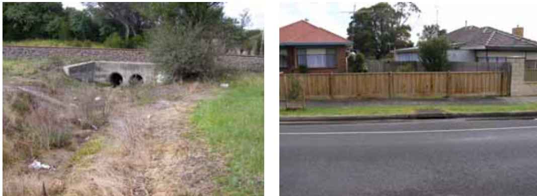
Photos 9 and 10 Watsons Road Drain culverts under Railway and looking downstream to the blocked flowpath from Waterloo Road in the Mervyn Street/Desmond Street subdivision.
