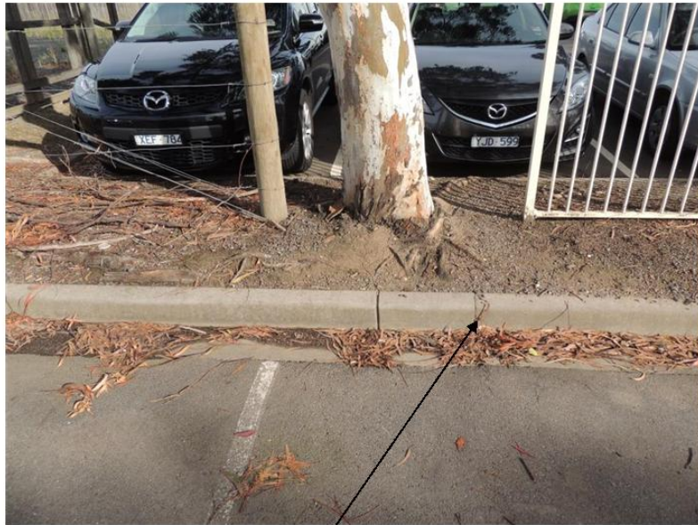
Curb damage by tree 10
