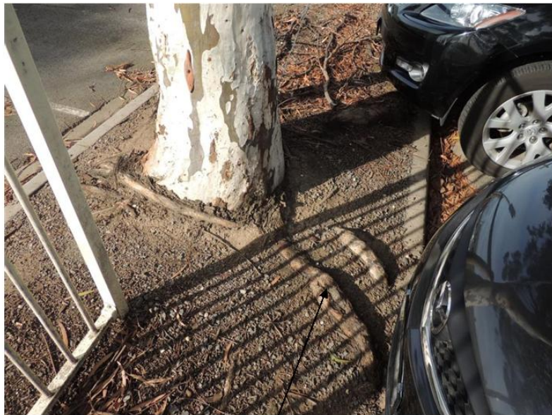
Surface and girdling root
