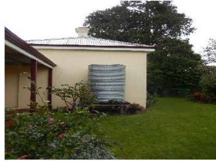
Rain Water Tank
