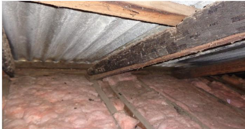
Re-enforced Fire Damaged Rafter
