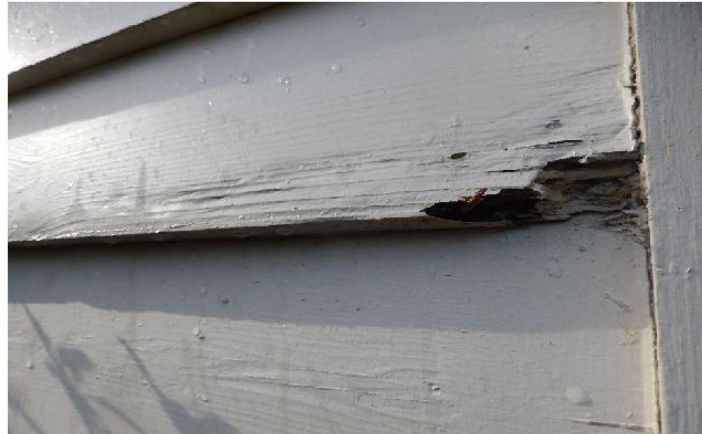
Weatherboards – Dry Rot (Western Wall)
