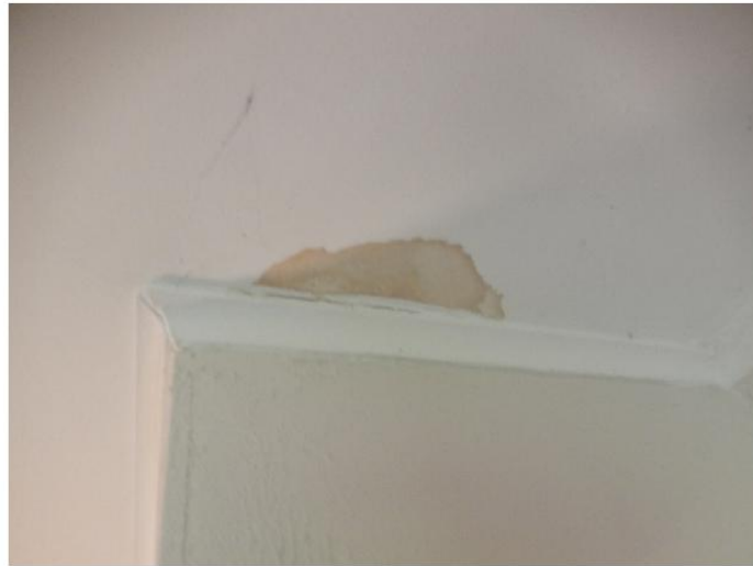
Ceiling Water Mark- Villa
