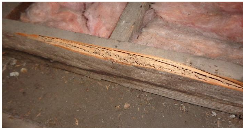
Termite Damaged Ceiling Joist
