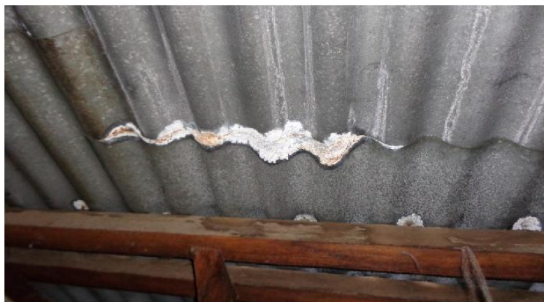
Roof Cladding – Corrosion
