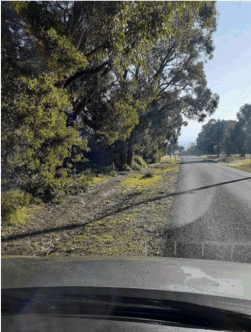
Uneven pathway with declines that fill with water causing deep mud holes.
