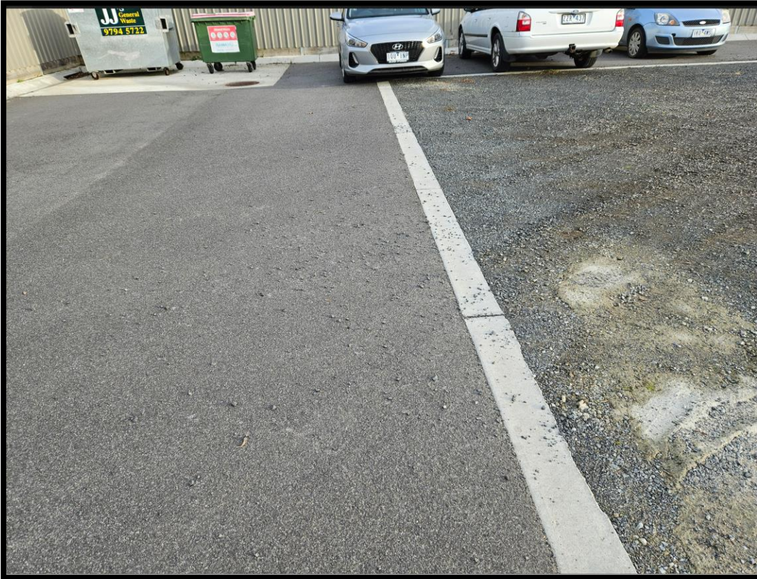
Construction of access, access to 24, 26 and 28 Buckley Street and construction of concrete foundation under bins
