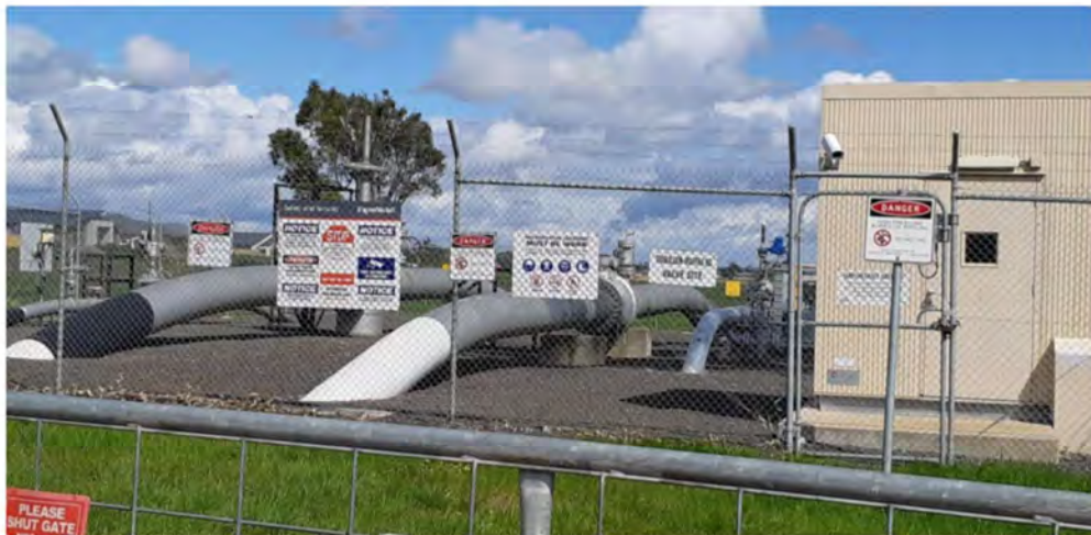
Plate 2: High pressure buried oil pipeline compound in southeastern corner of the site
