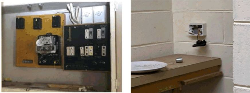
Figure 5 Pavilion Meter Box and Damaged Power Point
