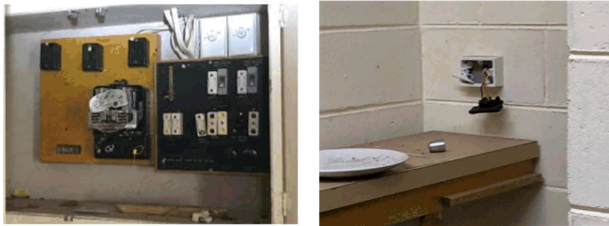
Figure 5 Pavilion Meter Box and Damaged Power Point
