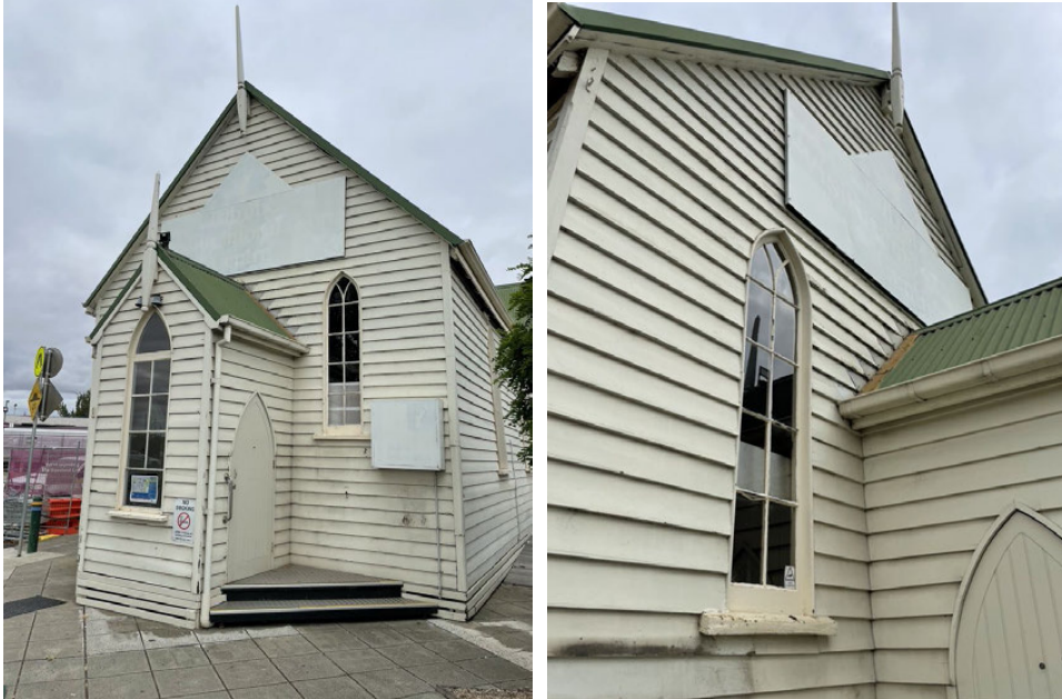
Views of the front elevation showing the reconstructed porch and finials, as well as the signboard covering one of the circular gable vents
