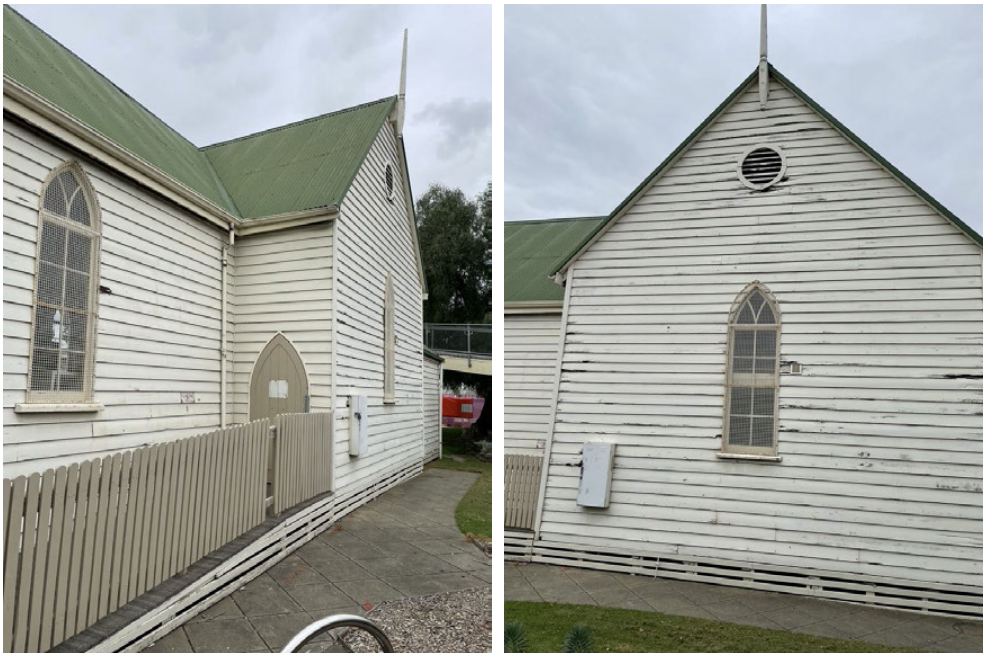
Views of the west side, note typical circular louvred vent in gable end (note visible deterioration to weatherboards at wall corners in the image at right).
