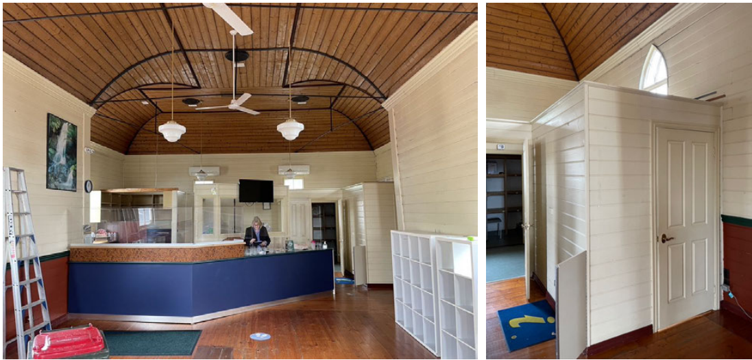
At left, view looking toward the rear showing the non-original counter and partitions installed for the Visitor Centre use. At right, toilet addition.
