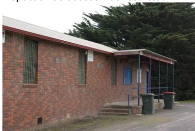
External access appears not compliant to current BCA / DDA requirements.
