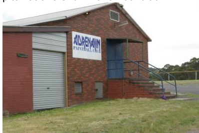
Football Oval Pavilion – no internal inspection as access was restricted. External access appears not compliant to current BCA / DDA requirements.
