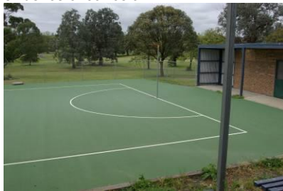
Netball Court appears in a good condition. Would recommend colour the 'safety runoff' area around the court a different colour to minimise confusion.
