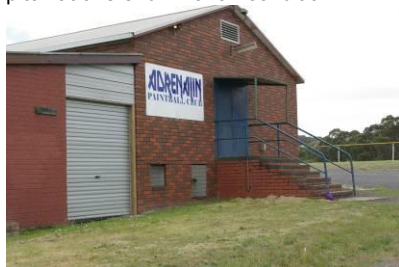
Football Oval Pavilion – no internal inspection as access was restricted. External access appears not compliant to current BCA / DDA requirements.
