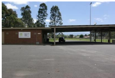
Soccer Pavilion – no internal inspection as access was restricted. Extensive covered area from pavilion to side of soccer pitch.
