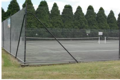
Tennis courts – asphalt/concrete courts. All appear in a fair condition with evidence of wear and tear and expansion cracks between courts.
