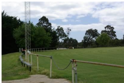
Boundary fencing and existing sport lighting towers appear 'tired' and have evidence of corrosion.
