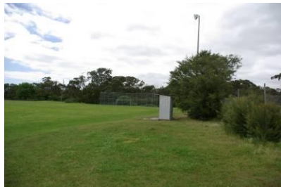
Goal end safety fencing to secondary pitch at one end. In a fair condition.
