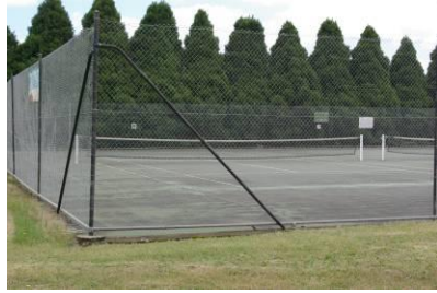
Tennis courts – asphalt/concrete courts. All appear in a fair condition with evidence of wear and tear and expansion cracks between courts.
