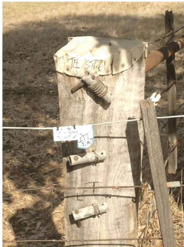
Photograph Four: Existing Telstra connection for 76 Stuart Street on western side of road.
