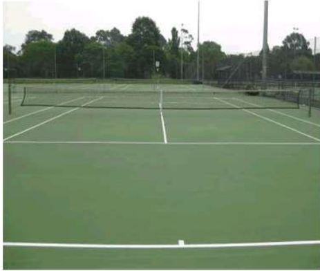
1. Typical view over tennis court # 3 – acrylic 'Laykold' top over original 'Rebound Ace' Synpave court.
