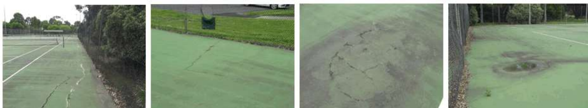
There are many examples of the court pavements failing and collapsing throughout all court enclosures.
