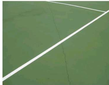
10. New tensile cracking to Court # 15 following seismic event.
