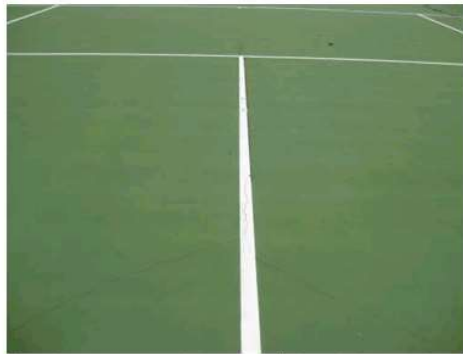
9. Long term crack on court # 6, existing crack has propagated further following the seismic event.
