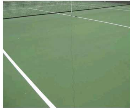
8. New tensile cracking to Court #3 following seismic event.
