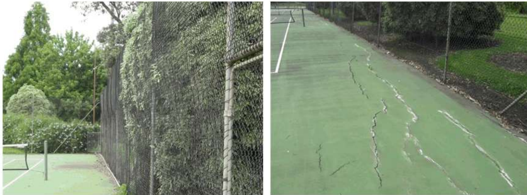
Large trees and shrubs are just too close to the courts. This creates pavement problems, adds stress to the fencing and increases the amount of debris on the courts. Pavement failures are often a result of interference from trees.
