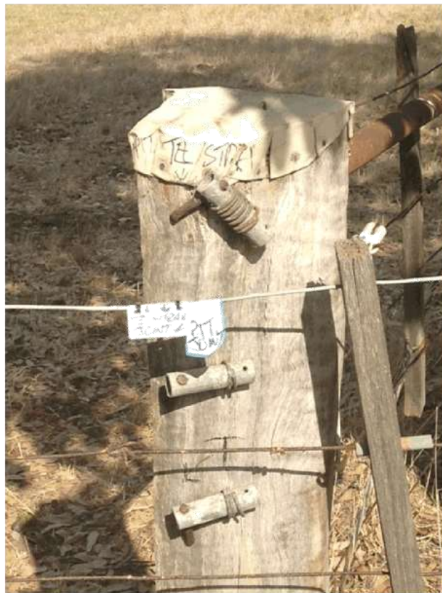
Photograph Four: Existing Telstra connection for 76 Stuart Street on western side of road.
