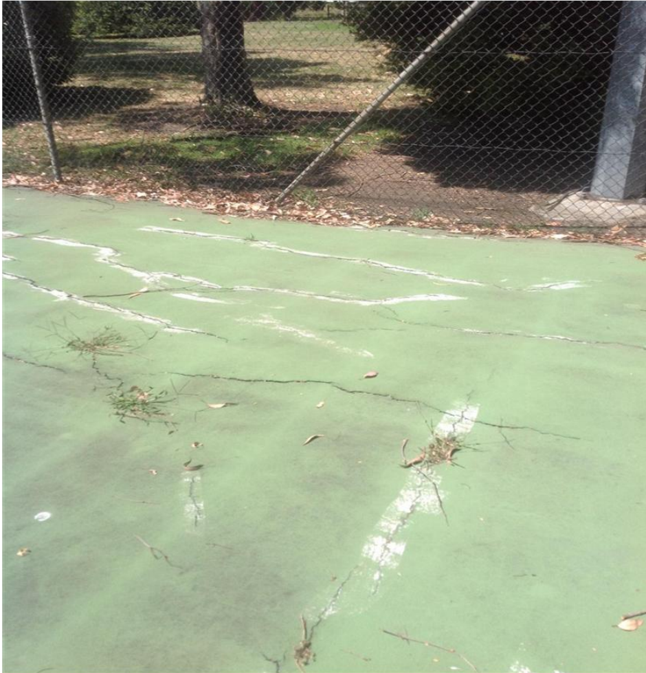
Evidence of past crack repair attempts and further new cracking throughout the court can be seen above.
