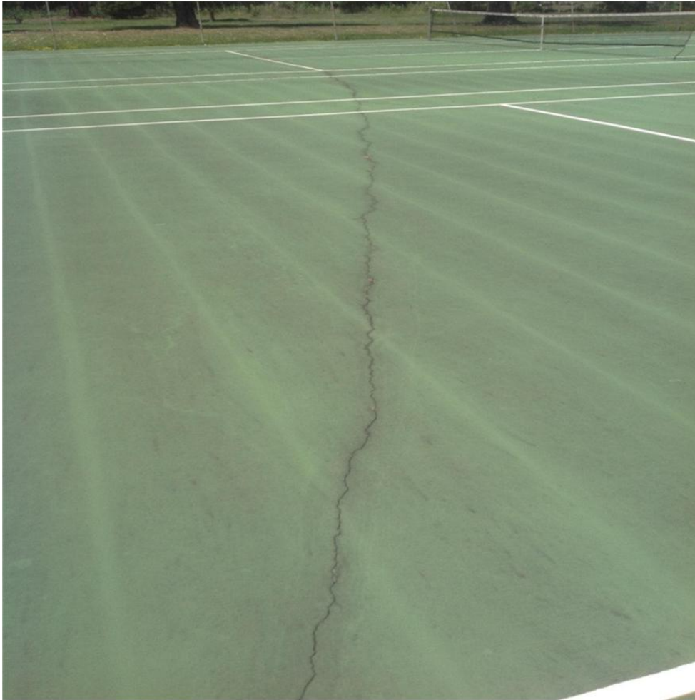
The cracks that have now appeared throughout the pavement (which were not evident in 2011) stem right across numerous courts and each and every court enclosure.
