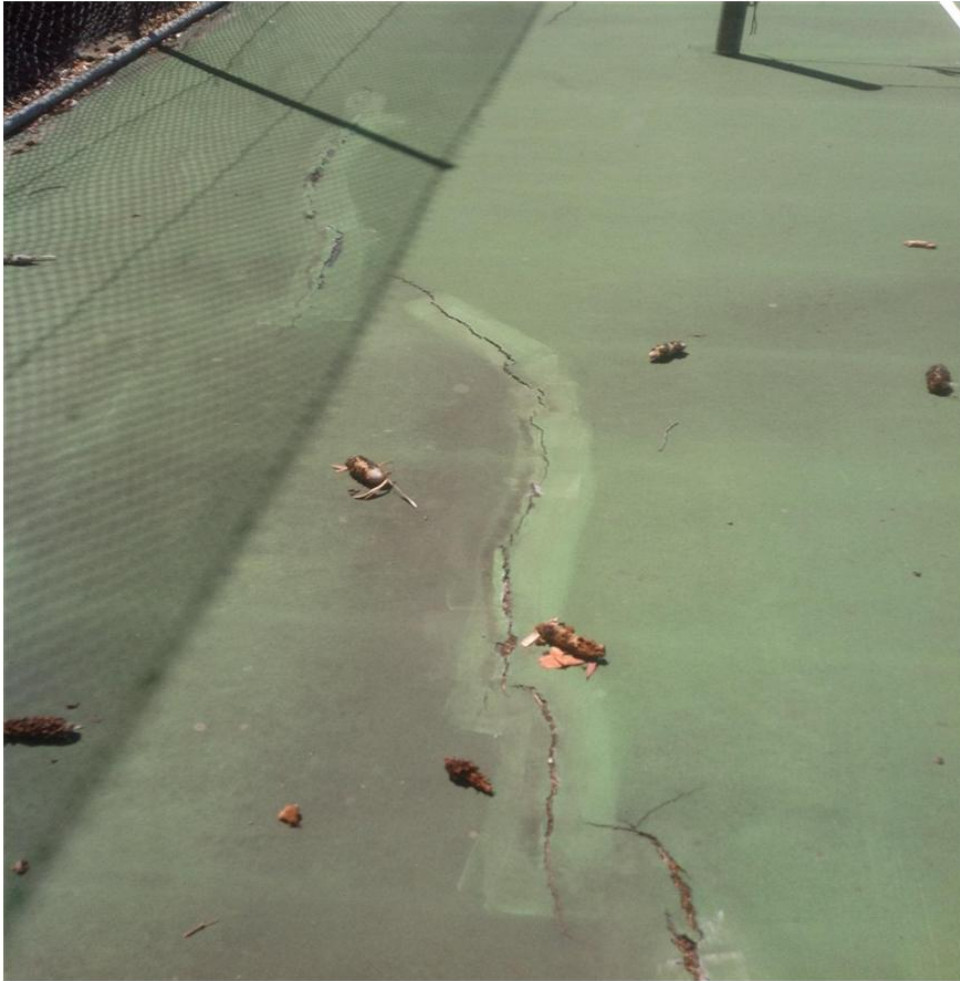
More pavement collapse where the pavement is situated close to a large Banksia Species. Not only do the roots undermine and damage the courts, the leaf and seed pod shedding also damages the sports surface and makes the courts unsafe.
