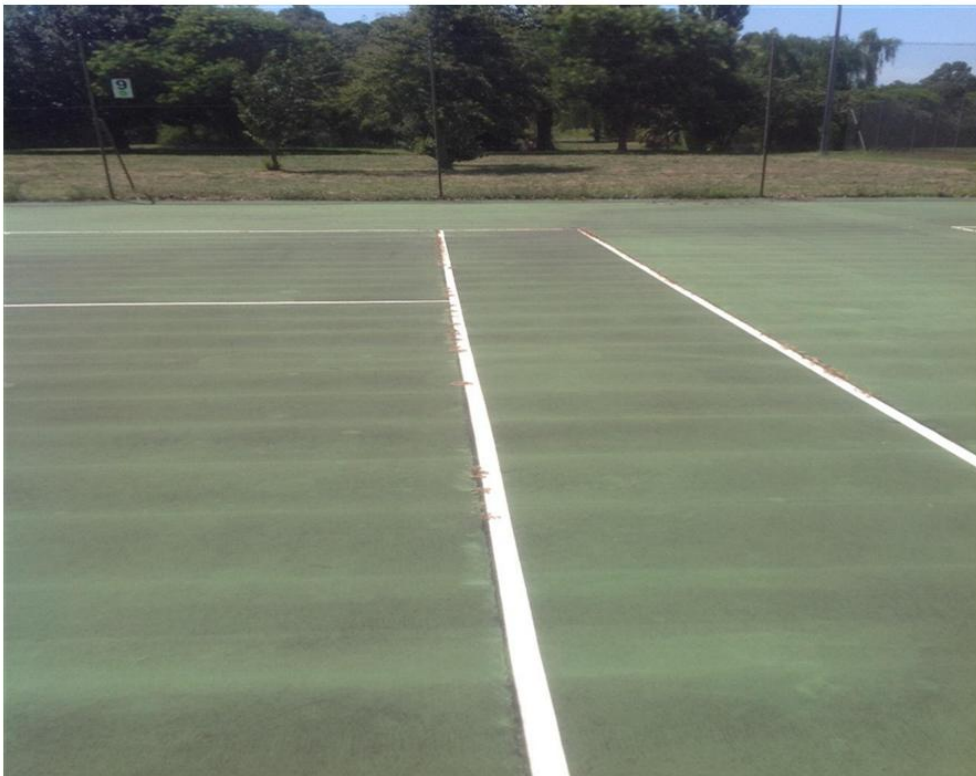
The picture above shows opportunistic weed growth within the cracked asphalt directly along the tennis court lines.
