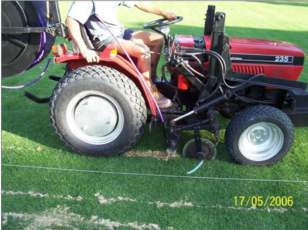
Figure 3. Photo of typical subsurface irrigation installation from Netafim brochure. Note the cutter wheel making a narrow slot for the pipe that rolls off the drum and is inserted below the surface.
