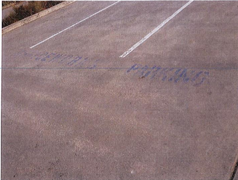
Figure 15: 'Officeworks Parking' signage
