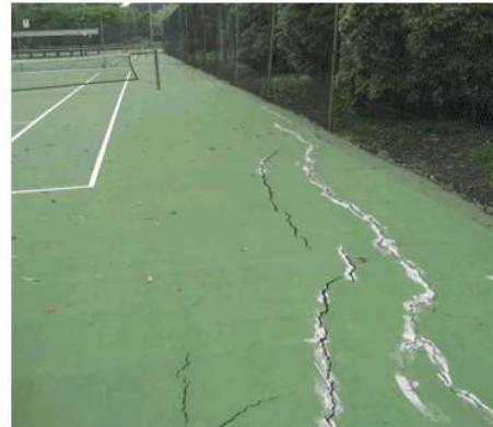
2. Looking west along northern boundary – long term cracking caused by adjacent trees.
