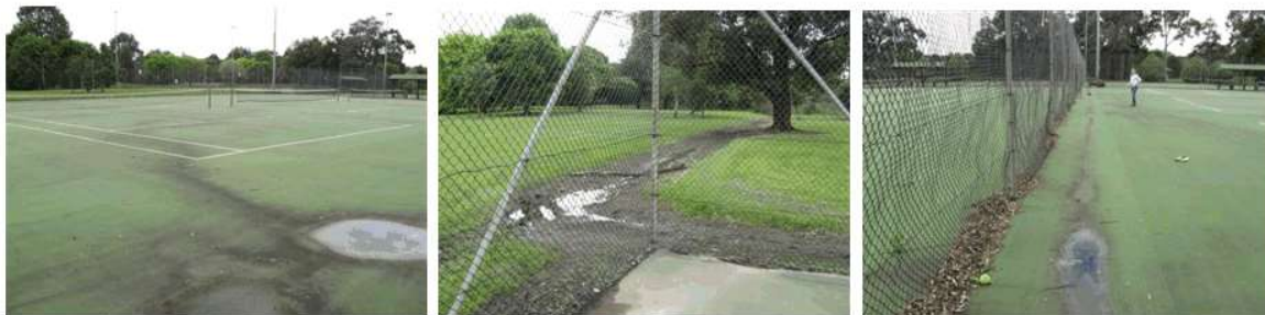
Drainage is a major problem at this site, both within and outside the court enclosures.
