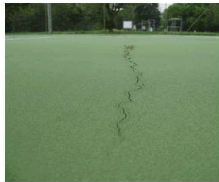
4. Typical long term cracking to courts – note weeds in crack.
