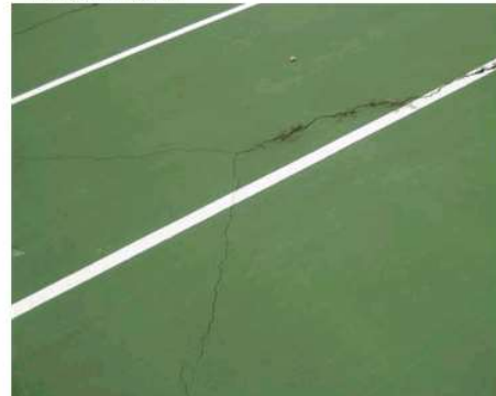
6. Long term crack on court # 7, existing crack has propagated further following the seismic event.
