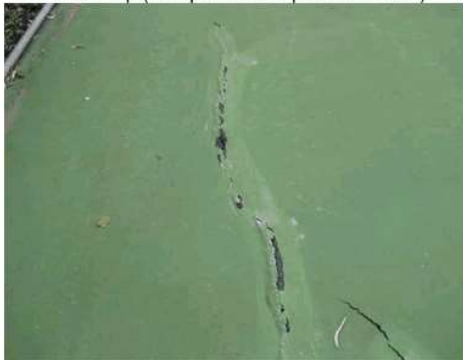
5. Long term cracking to north edge of courts – past repairs evident – a combination of tree root activity and differential shrinkage of clays.
