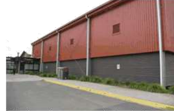
Existing show court exterior. Sub floor venting is restrictive due to levels of landscaping and entry path.
