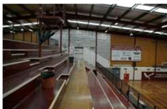
Seating plats appear too narrow and too high. Main circulation path (centre) should be provided a handrail to minimise any fall risk. Balustrade to edge not compliant – appears to be less than 1.0m in height. Also can be climbable.
