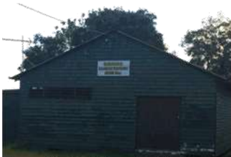
Pigeon Club building. Aged facility needing refurbishment
