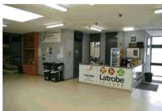
Main entry, control / reception counter. Counter not catering for wheel chair access by patron/ player.
