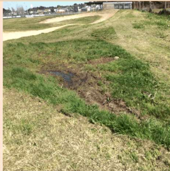
Image 9 – Inadequate drainage near track – Ronald Reserve, Morwell
