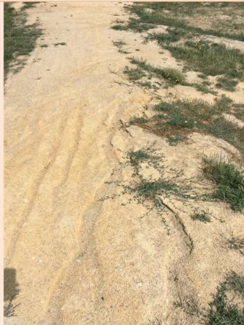
Image 3 – Close up of erosion on riding surface caused by draining water at Glendonald park, Churchill
