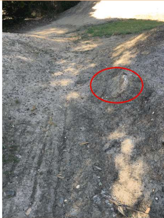
Image 5 – Large piece of concrete with steel rebar protruding at Yallourn North BMX track. Note: This large piece of concrete has been removed however it is likely that similar material is contained within the BMX tracks but remains unexposed at this time.
