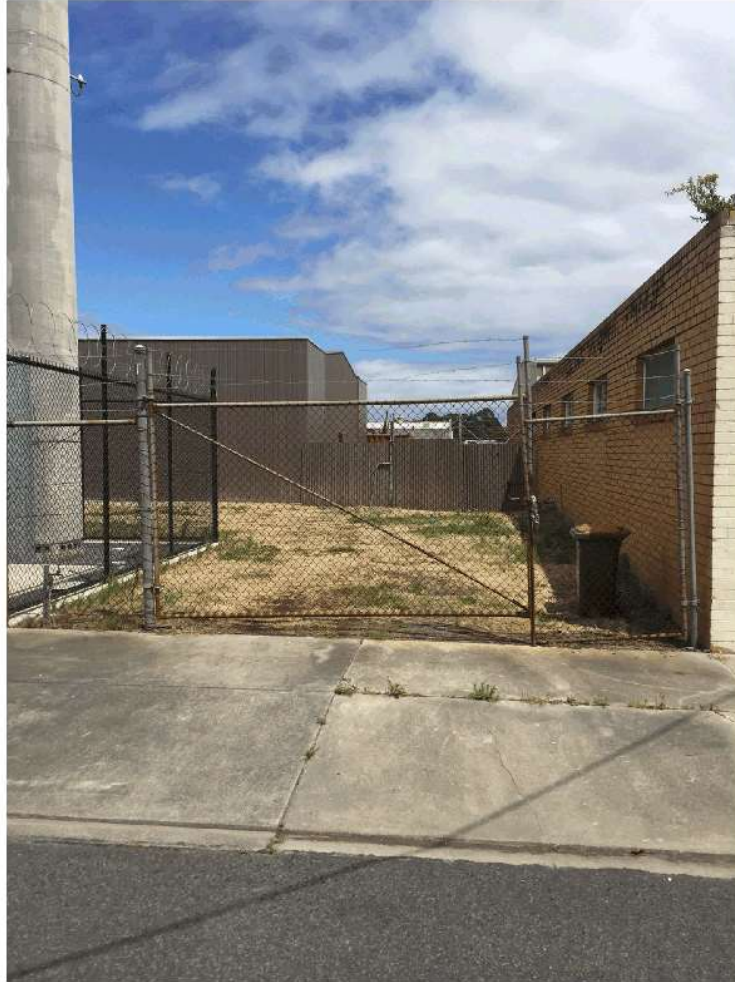
Photograph 1: Discontinued laneway to be transferred to the owner of 2 Short Street, off Collins Street. Brick wall at the rear of 31-33 Shakespeare Street shown on the right side.
