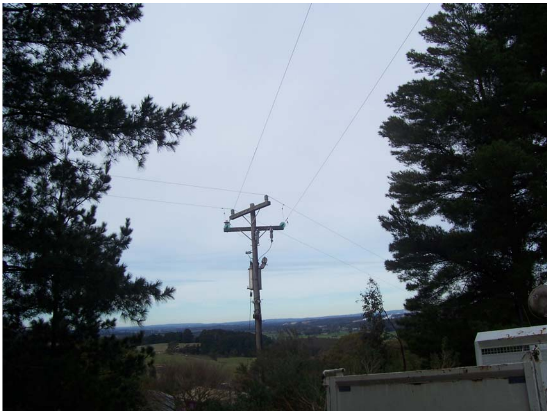
The above picture shows the power line that runs in the private paddock on the east side of the trees.
