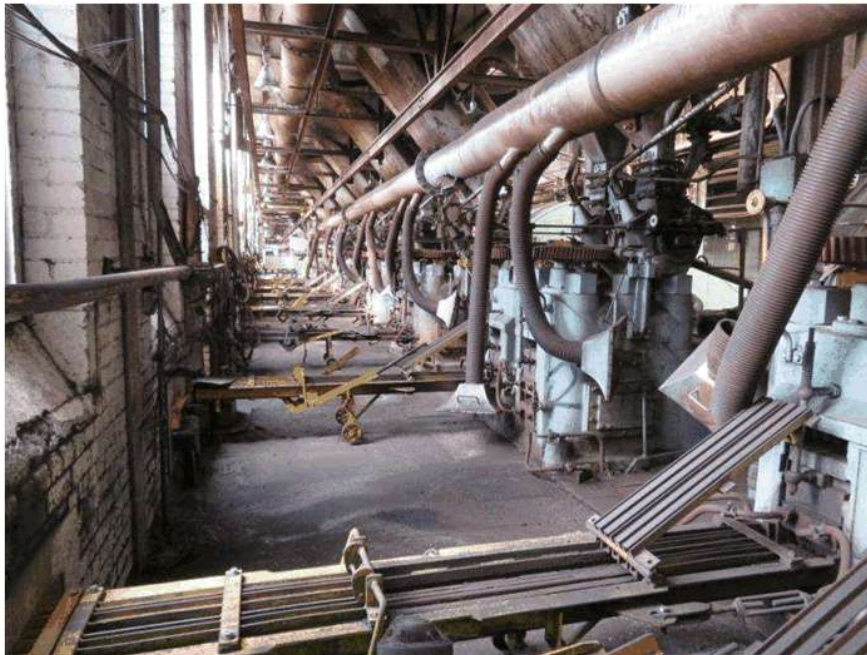
View of conveyors leading from briquette machines to external conveyor, looking east.
