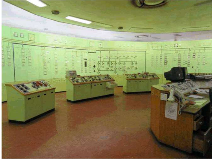
View inside the Power Station Control Room.
