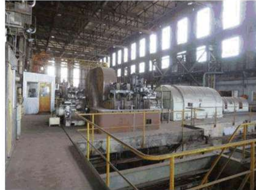
Power Station Turbine House
