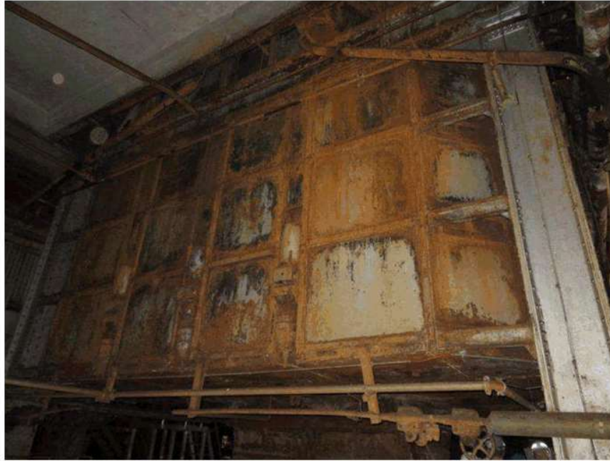
Brown coal fired boiler inside the Power Station.
