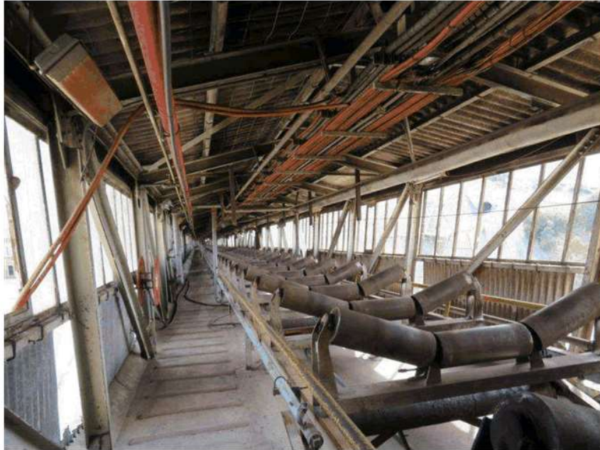
View of the conveyor from North West Corner Station to No.1 Briquette Factory.
