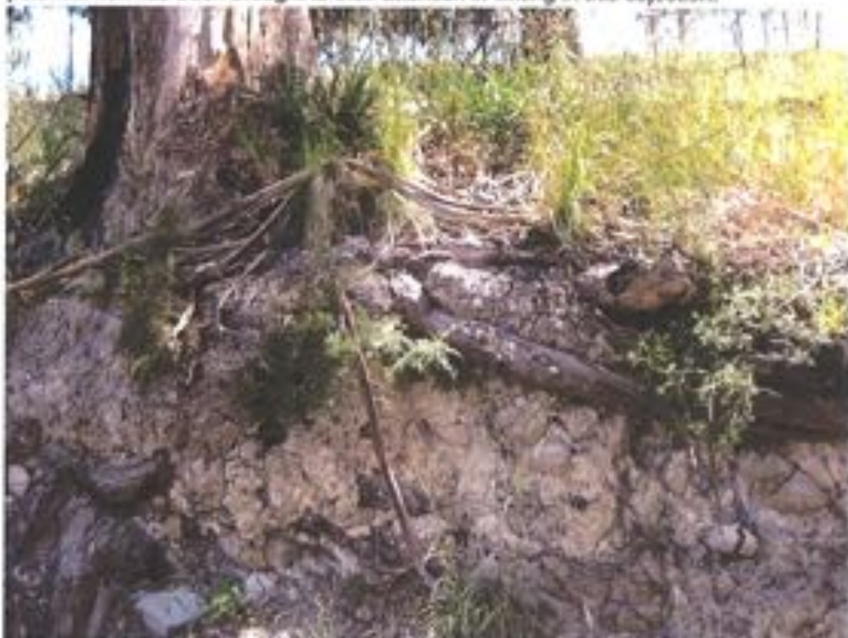
Photo 4: One of the Eucalypts to be removed – note tree root interlock to underlying soils providing slope stability. Tree removal will remove this stability.
