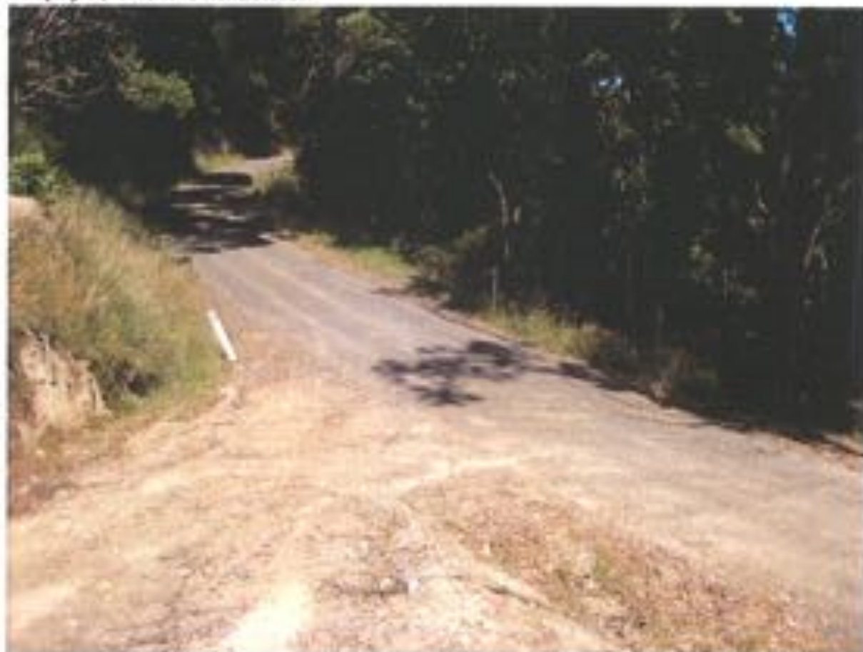
Photo 6: Jumbuk Road past Jumbuk Hall, logging road installed with no crossing, drainage causing road to wash away- demonstration of lack of care of Councils assets.
