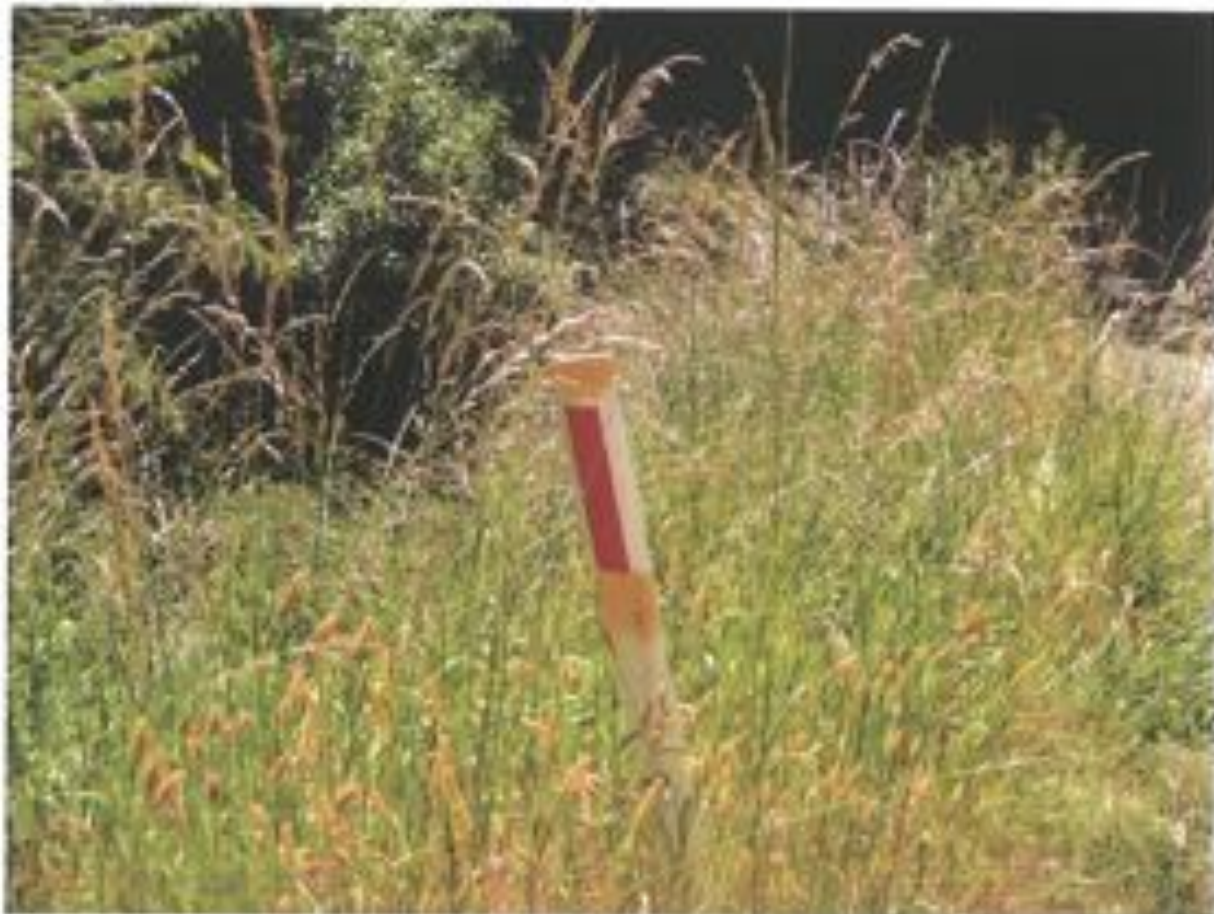
Photo 5: Jumbuk Road past Jumbuk hall, past internal corner collapse not repaired – yellow paint indicates caution for contractors – demonstration of lack of commitment to repair of damage caused by their vehicles.
