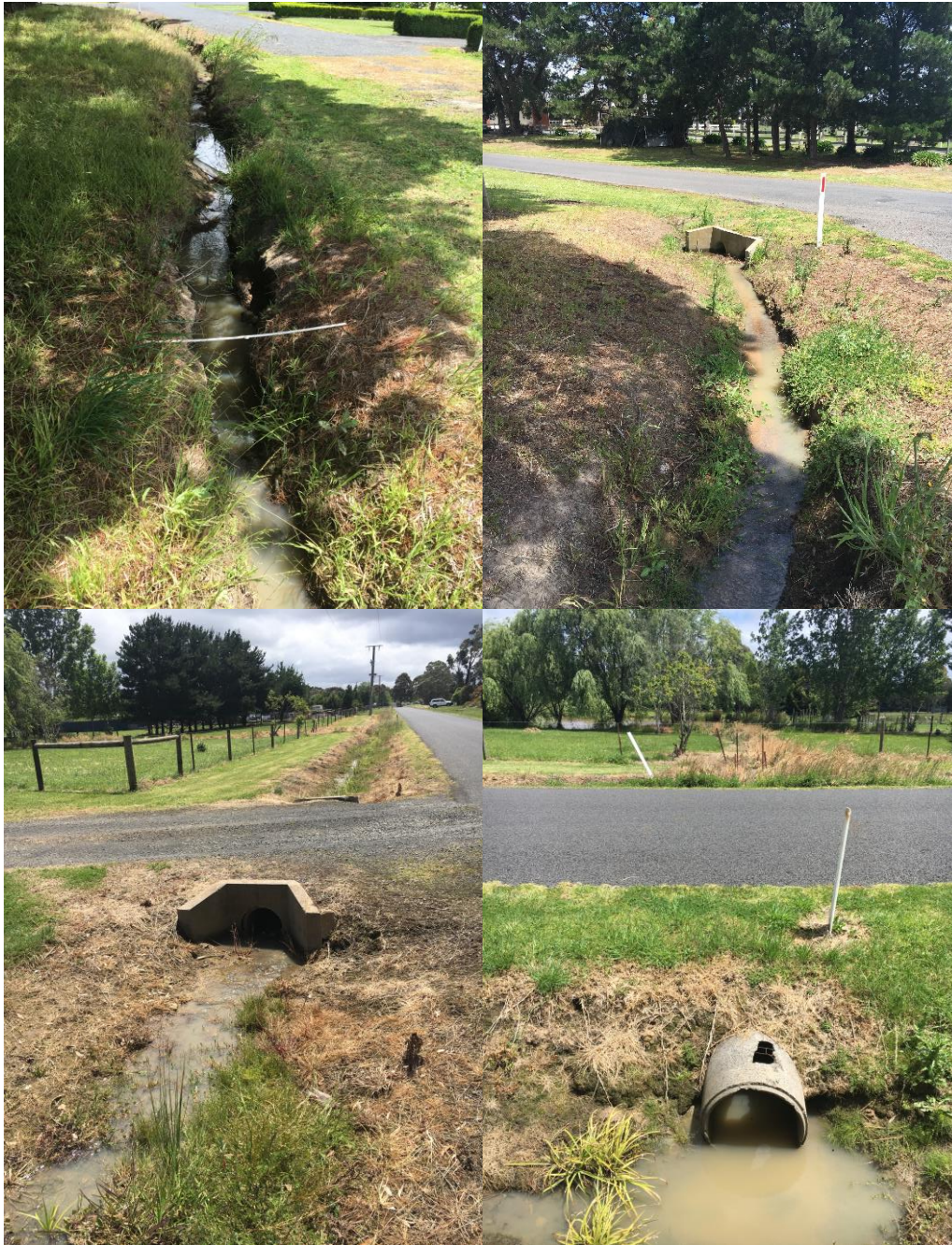
FIGURE 4-1 TYPICAL DRAINAGE CONDITIONS IN JASON STREET
