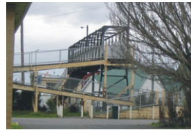
Poor pedestrian connection over the railway line
